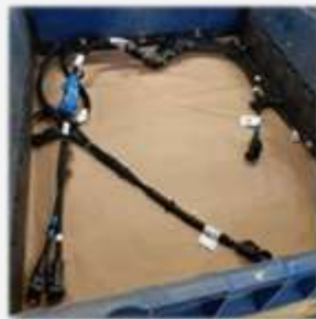
Figure 10. Battery cable harness.
